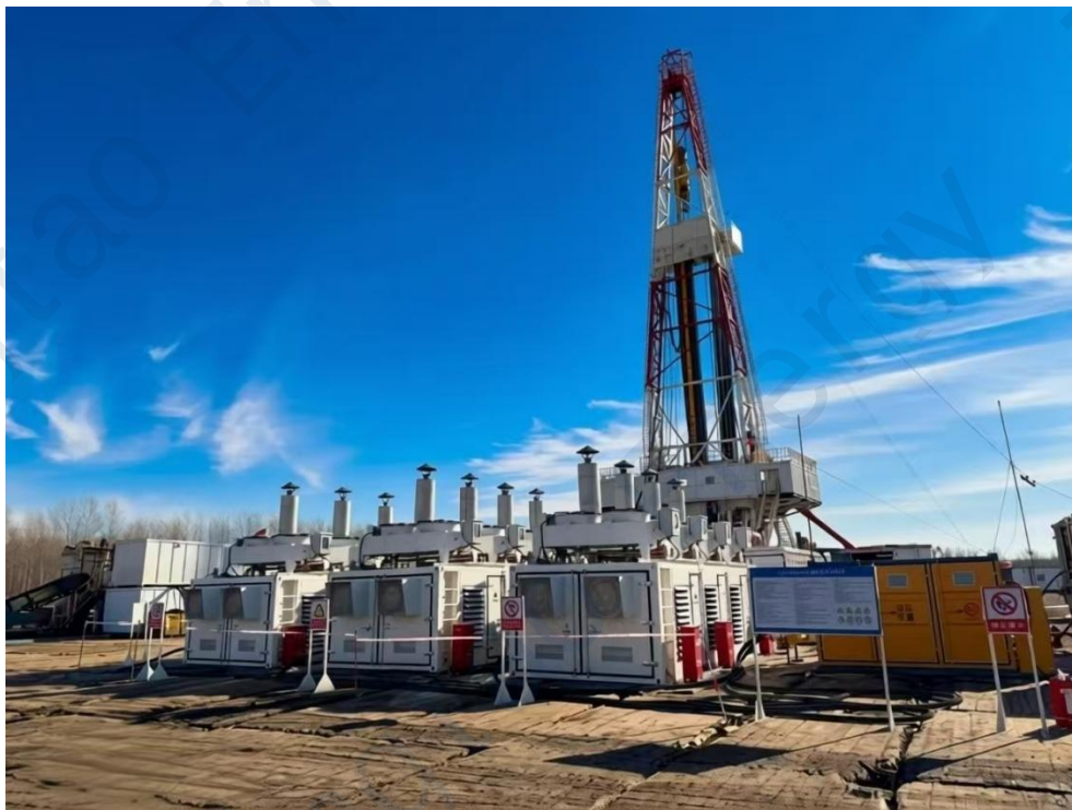
Fig. 4-1: Integrated Power Generation System for Drilling Rigs – Multi-unit Parallel Operation in Oilfield Conditions.
