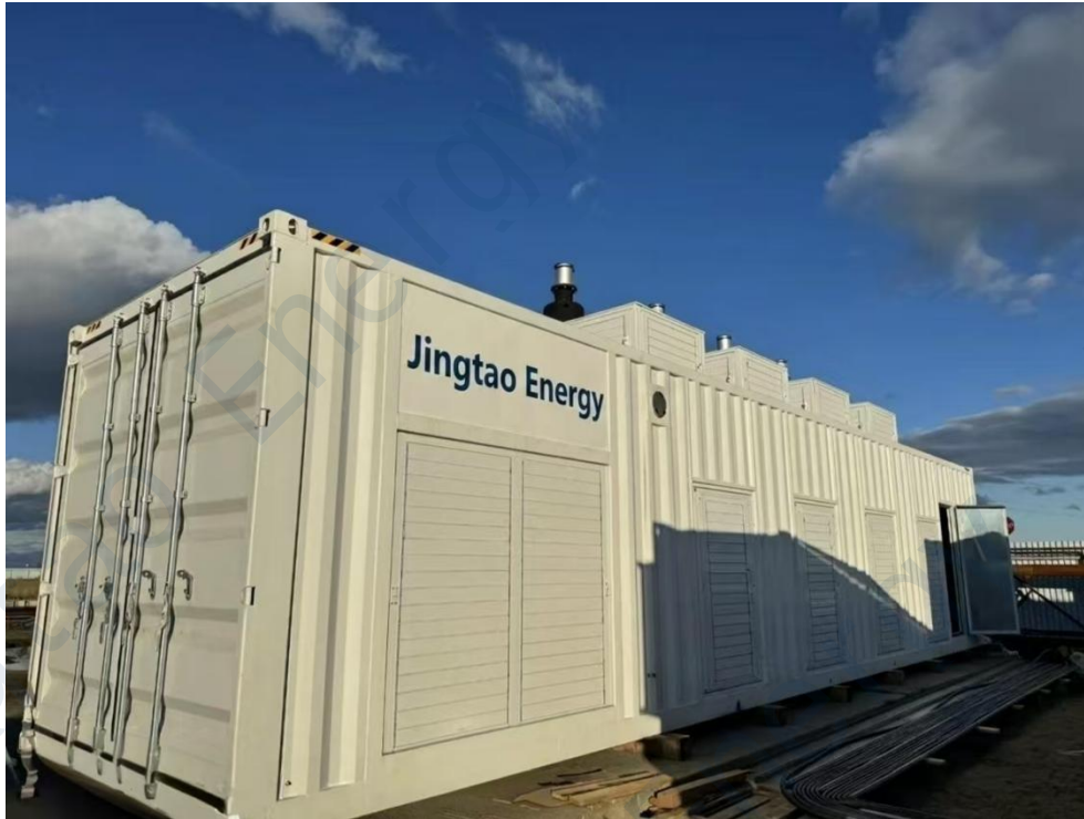
Fig. 2-1: Jingtao Energy CHP System - Designed to tackle the challenges of associated gas utilization.
