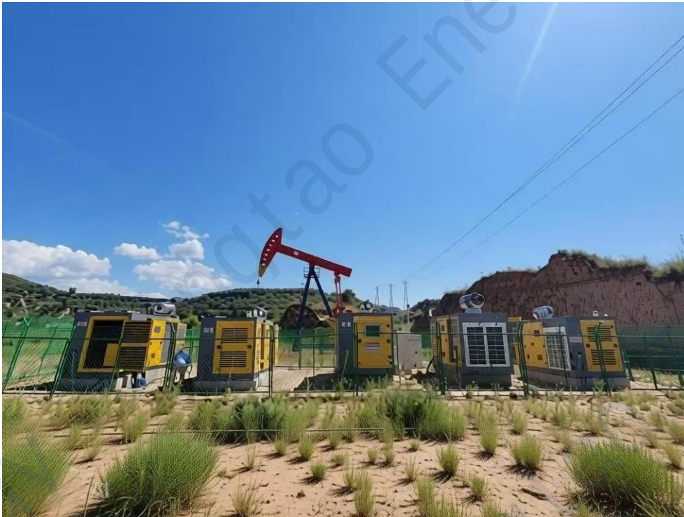
Fig. 4-2 Associated Gas Power Generation at Pumping Unit Sites – Turning Wasted Gas into Electricity.
